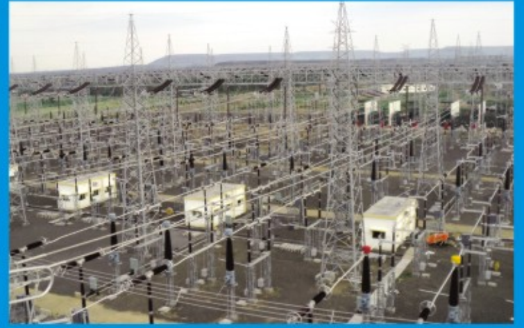
400 kV AIS at Lonikand, Maharashtra
